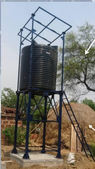
Water Storage Tank 5000 Ltr.
